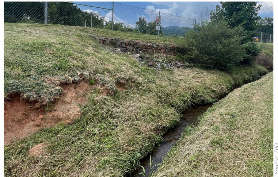
Image 37. Erosion along Bumgarner Branch Creek
